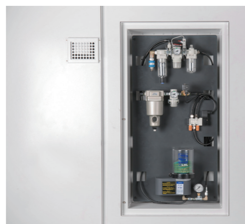
Through centralized management of pneumatic solenoid and lubrication pump, it made the daily maintenance easy.
